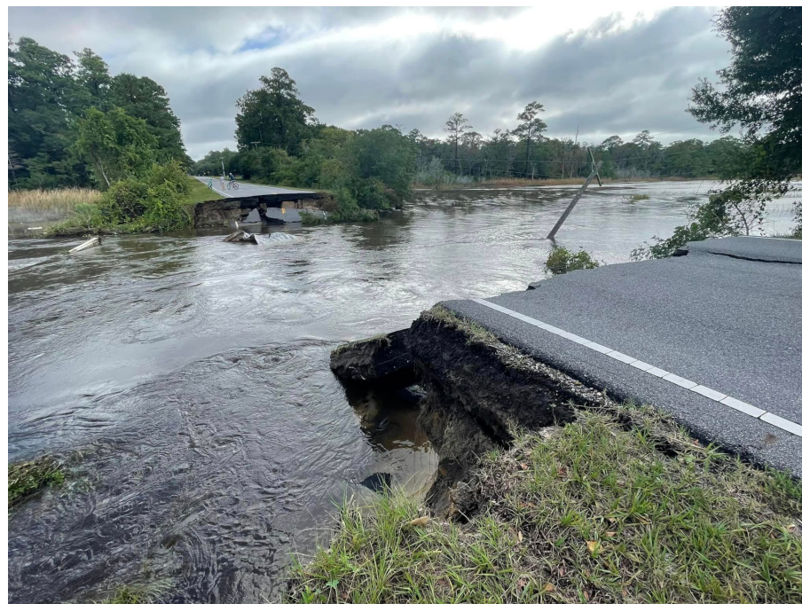
East Moore Street washed out (Southport Police Dept.)
